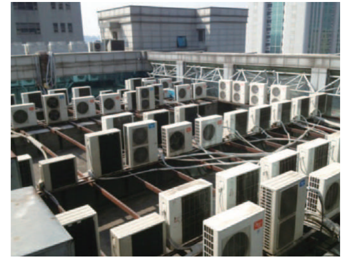
Before Multiple brands installed
