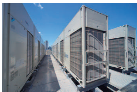
VRV Q installation
