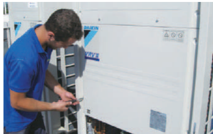
Thirty-nine VRV III-Q units serve 215 cassette type indoor units and 35 VAM ventilation units.
