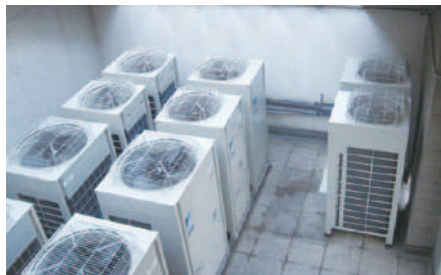
The original VRV units that ran on R22 were replaced with VRV III-Q units running on R410A.
