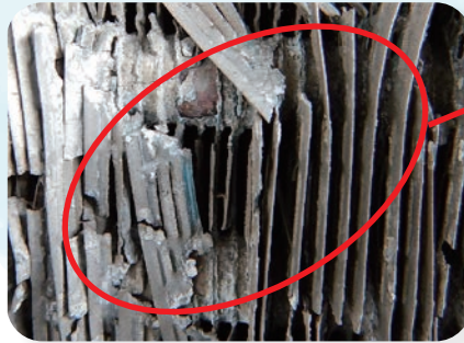
Inadequate Cooling Performance
