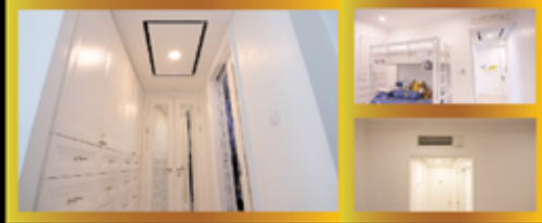
Project Pakubuwono Residence ( Jakarta ) Designed by LAnD Studio AC Installed by Daikin Proshop AC System VRV HS + Single SkyAir
